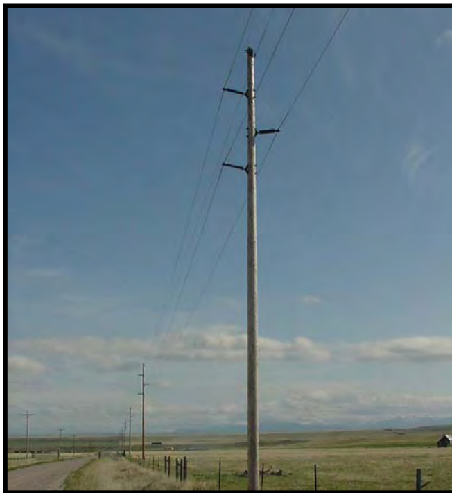
FIGURE 8-B. Photo of typical 69kV vertical wood pole construction similar to the Project 69 kV transmission line. (photo does not include 7.2 kV under-build)
