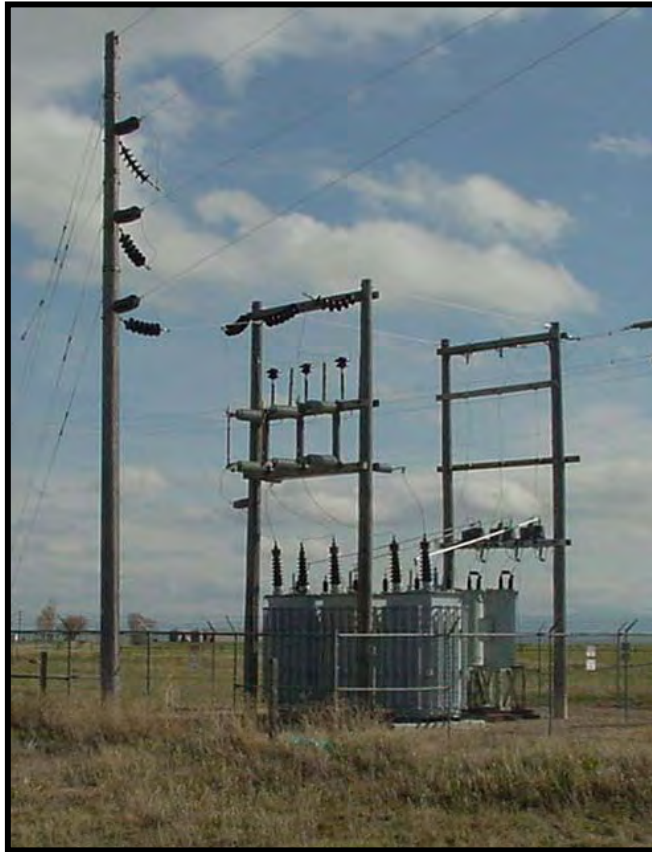
FIGURE 8-A. Photo of typical substation similar to the Project substation to be located approximately four miles east of the Forest Boundary.
